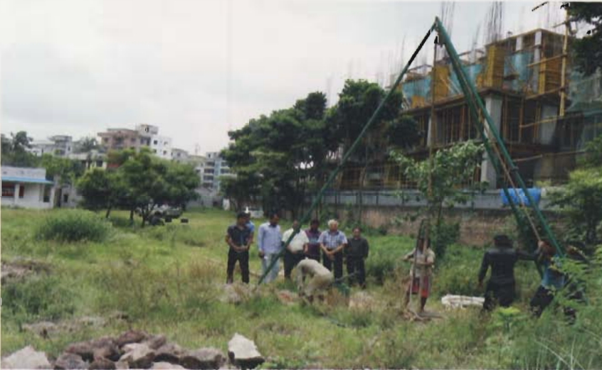
Vice Chancellor Dr. Profulla C. Sarker along with others watching the beginning of construction work at the permanent campus of the University
